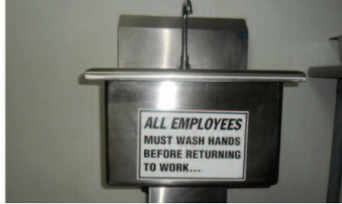
Hand wash sink with sign
