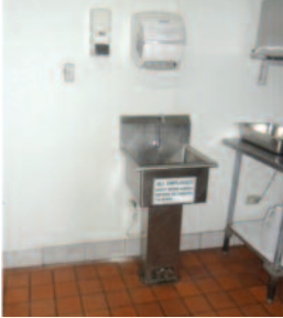
Hand wash station
