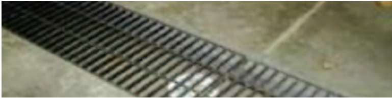
Figure 7: Open drains with suitable cover to prevent entry of rodents
