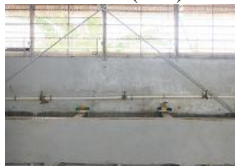
Concrete wash tank
