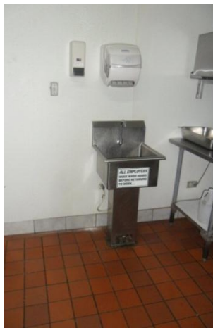
Hand wash station
